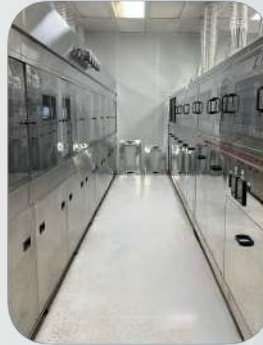
MACHINES IN CLASS 1K CLEAN ROOM
